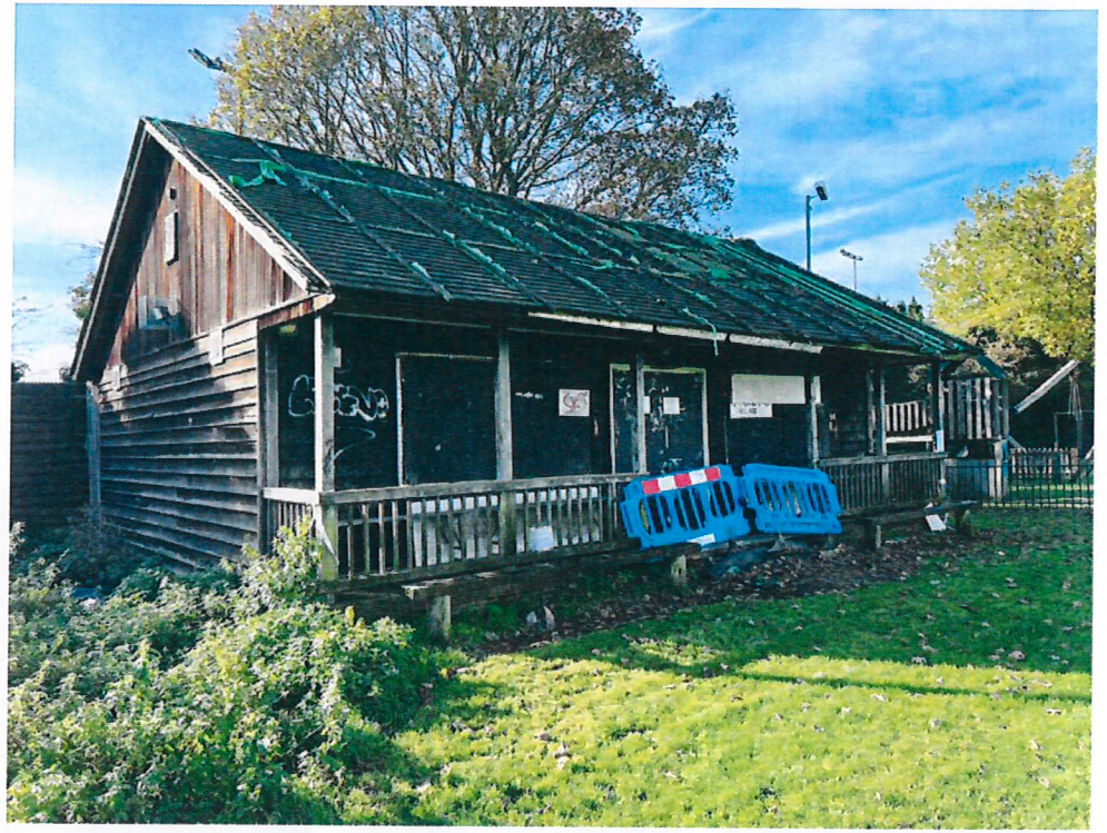
The now unused and unsafe Sutton Valence sports pavilion
